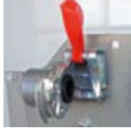
In-correct Application / Hatalı Uygulama
