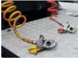
In-correct Application / Hatalı Uygulama
